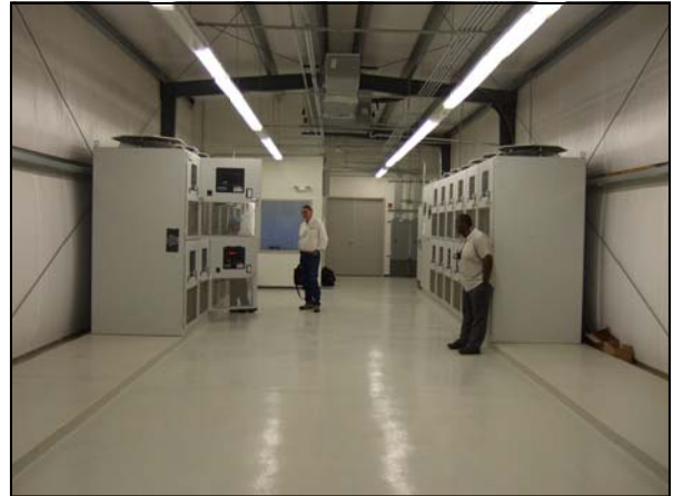
Pete Hackbusch shown inspecting the new switchgear style regulators at Southern California Logistics Airport New Lighting Vault designed by Dinter Engineering Co.
